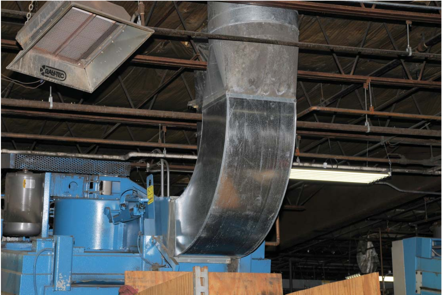
By installing a duct system with an outlet that went straight to the roof, Packerland enabled its dryers to ‘breathe.’
