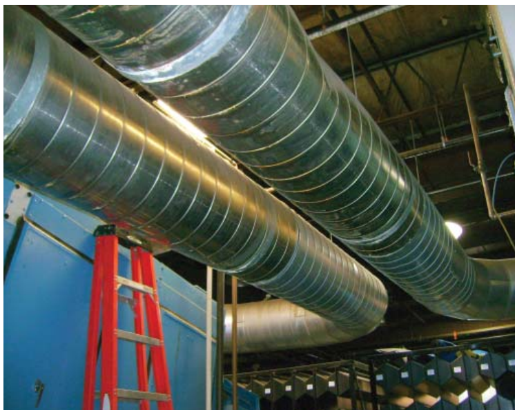
Another view of old duct system. Long runs like these reduced efficiency in the dryers.
