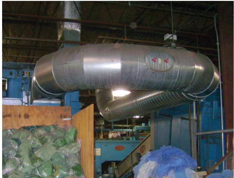
Shown above is the old dryer duct system with twists and turns that produced back pressure and slowed drying times.
